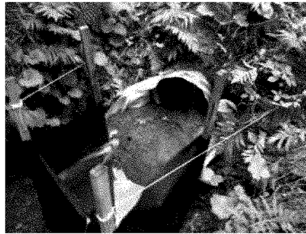
Figure 7: Silt fence constructed of plastic sheeting to retain sediment and filter fabric to pass stormwater, installed at culvert outlets to trap material eroded from roads and roadside ditches.
